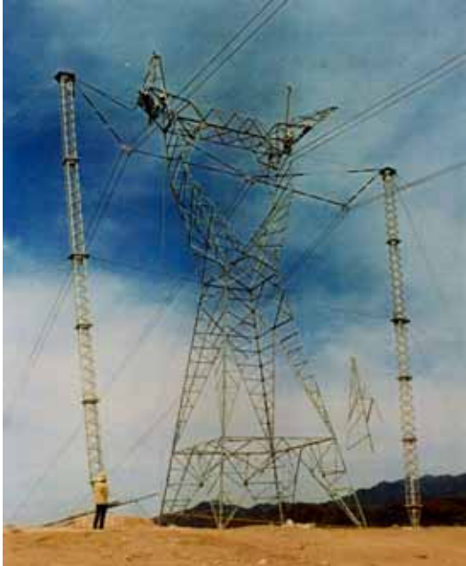
Chainette: This 400kV ERS is supporting the line during re-construction of the permanent tower.
