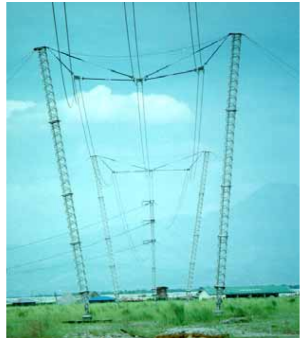
Chainette: These 230kV ERS were built for an emergency bypass and have been in service for 10 years.
