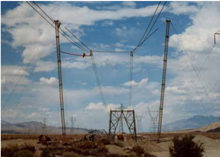
Sabotage of a critical 500 kV DC transmission line necessitated the erection of this Lindsey Emergency Restoration Structure. Total erection time was 5 ½ hours.
