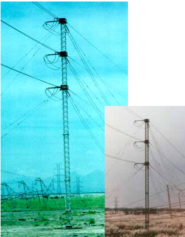
Vertical Three Phase Tension: This 230kV ERS In-Line Tension ERS was built after a major disaster. The picture above shows the same ERS 8 years later.
