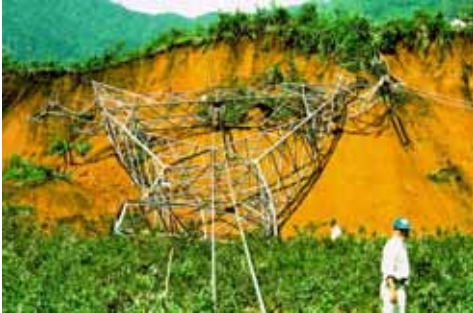
Hurricanes and mud slides caused this failure of a 400kV tower.
