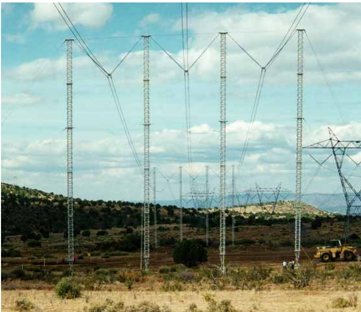
Four Column: These 500kV ERS are supporting the line while a substation is being built below it.
