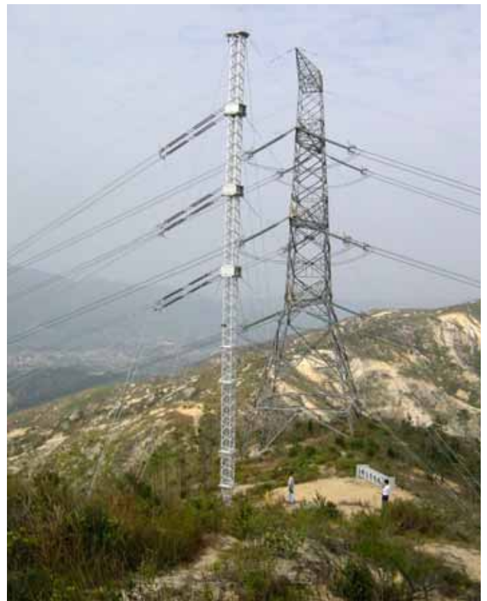
Vertical Three Phase Full Tension: This 400kV ERS Full Tension 3-Phase Dead End ERS was built as part of a bypass line. Note there are 4 subconductors per phase
