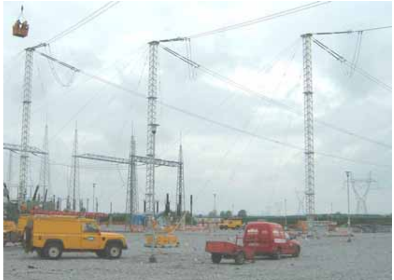
Horizontal 90 Degree Tension: These 400kV, 90 Degree Tension or Dead End ERS were built as part of a bypass during construction on the substation.
