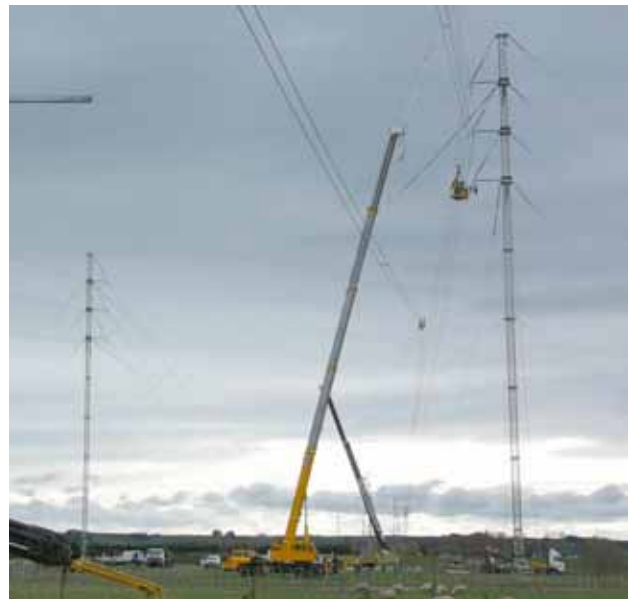
Angle Horizontal-Vee: These 220kV ERS were used to restore both circuits of a tower washed into a flooded river.
