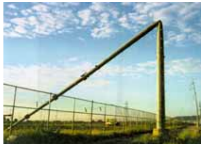
High winds and flying debris caused failure of this 115kV steel pole line.
