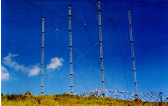
Four Column: This 400kV ERS was built in one day to support lines from a nuclear plant. Spans were over 800m on either side.
