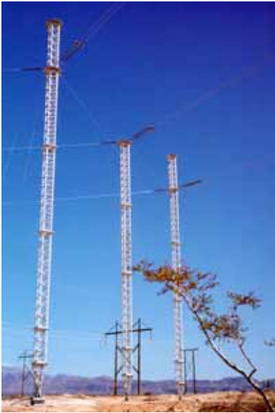
Horizontal 60 Degree Tension: These ERS Dead Ends were used to build a temporary 500kV bypass Line
