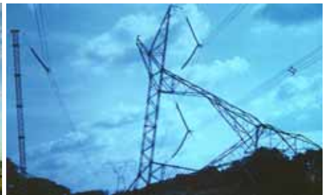
Dynamite charges toppled this 500 kV tower. A Lindsey Emergency Restoration Structure was used for a quick solution.
