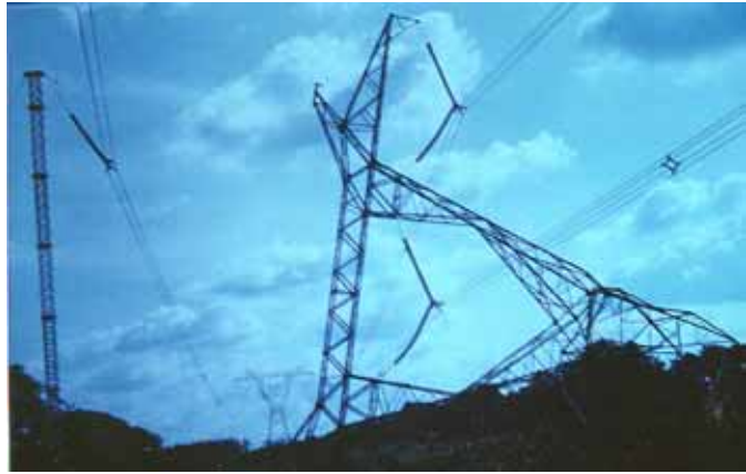
Single Phase Running Angle: This 500kV ERS was built to restore power after the permanent tower was sabotaged.
