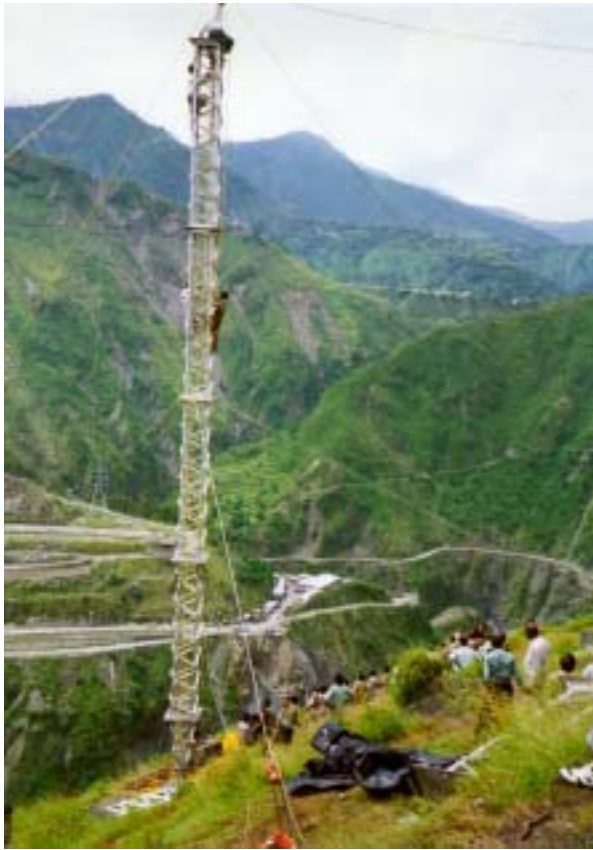
Figure 3 Erecting the bypass for Tower 59 using a Gin Pole and manpower to lift the ERS components.
