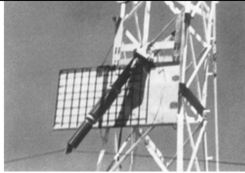
Figure 6. Tower No. 2 after test.
